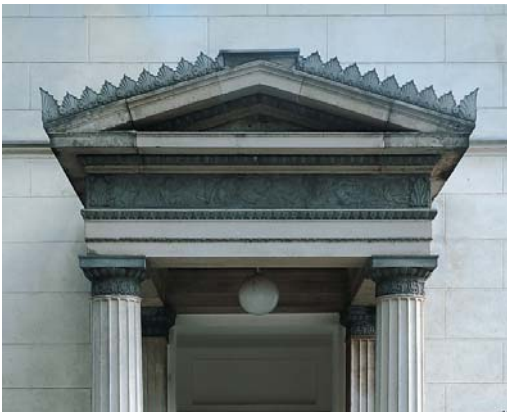
Fig. 7: Ornamental sheet-metal work at Schloss Glienicke, built by Karl Friedrich Schinkel between 1825 and 1828.
